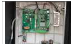
Control unit UNIGATE
